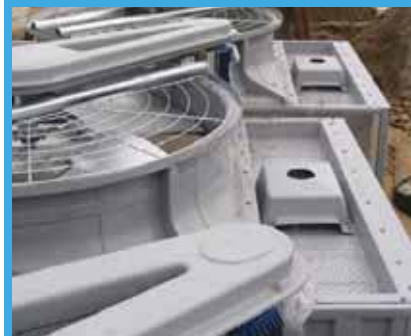
Hot Water Basin
